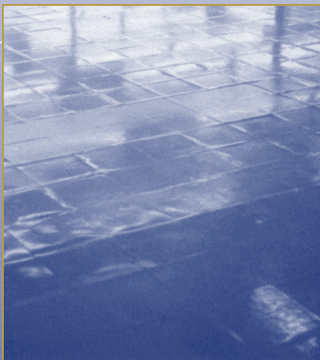
Alkaline salts can be carried with moisture to a floorcovering's surface, which can damage the floor and create a walking hazard.
