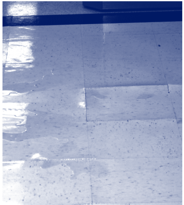
Buckled resilient tile installation.
